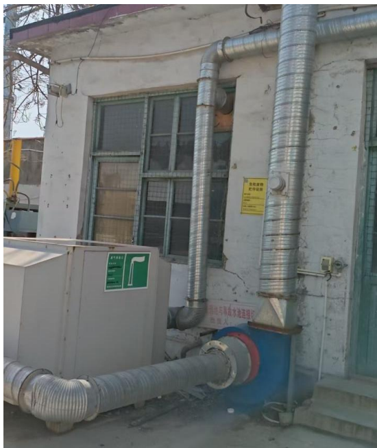
活性炭吸附装置+15m 排气筒 DA001
